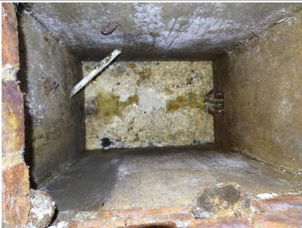
Manhole at front of property partially blocked
