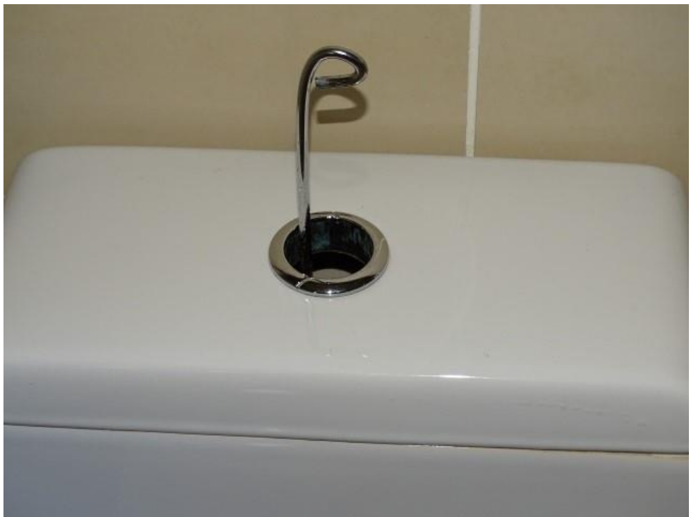
Flush mechanism button broken
