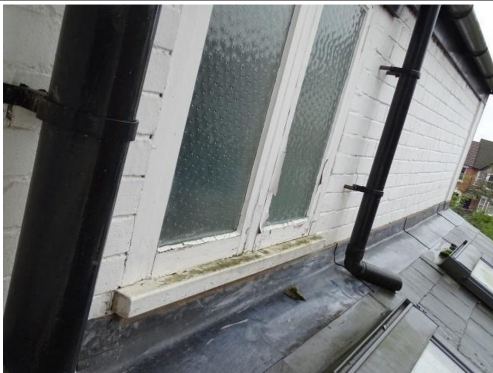
Bathroom fixed casement rotten
