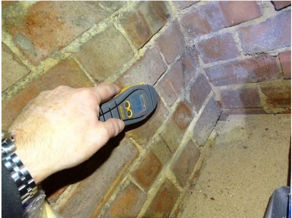
Wet wall in loft above bedroom 3
