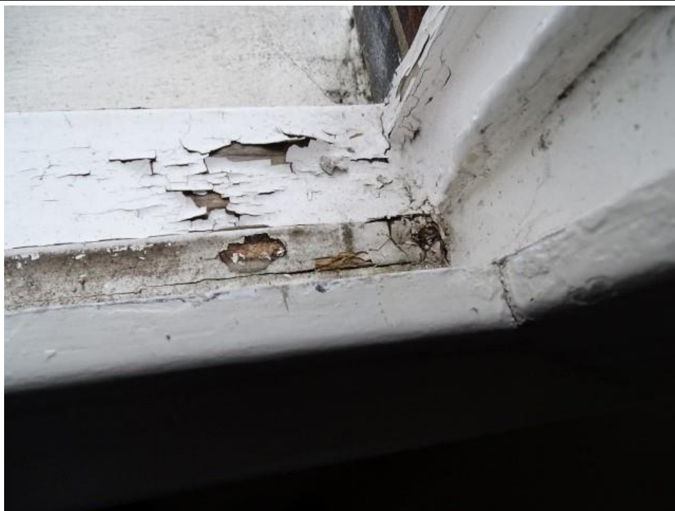
Bedroom 1 bottom sash frame rotten
